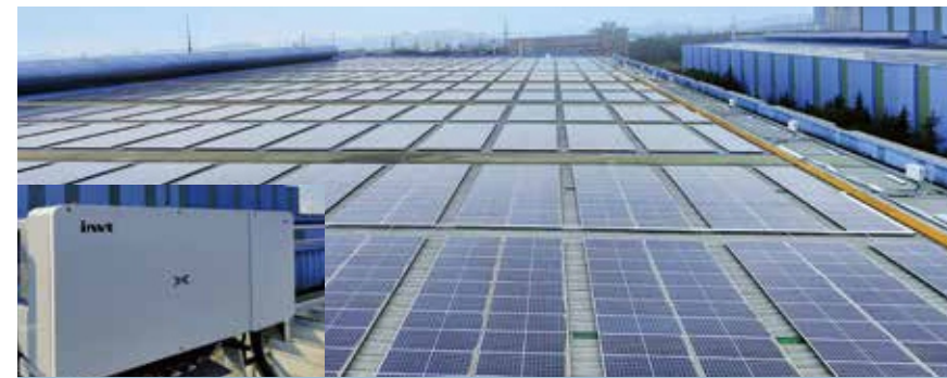
◆◆.◆◆MW Rooftop PV Plant in Hubei, China (XG◆◆◆KTR-X)
