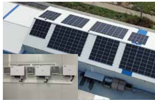
◆◆◆kW Rooftop PV Plant in Slovakia (XG◆◆KTR XG◆◆KTR)
