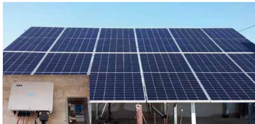
4kW Solar System in Israel (XG4KTR)
