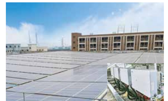
◆.◆MW Rooftop PV Plant in Guangdong, China (XG◆◆◆KTR XG◆◆KTR)
