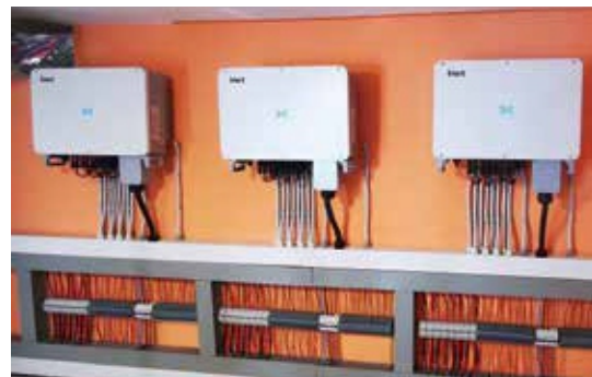
◆◆◆kW Rooftop PV Plant in Lebanon (XG◆◆KTR)
