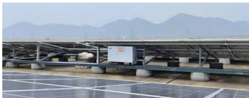
◆.◆◆MW Rooftop PV Plant in Hubei, China (XG◆◆◆KTR .XG◆◆KTR)
