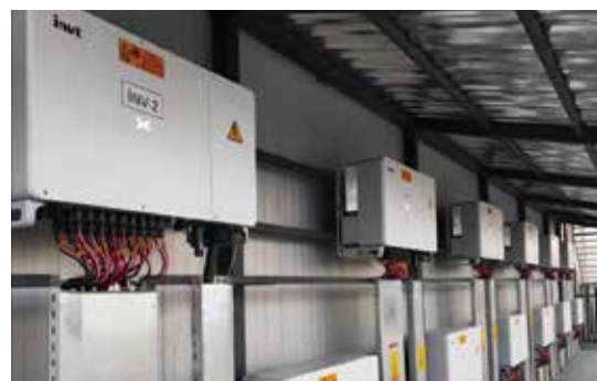
◆MW Rooftop PV Plant in Türkiye (XG◆◆◆KTR)
