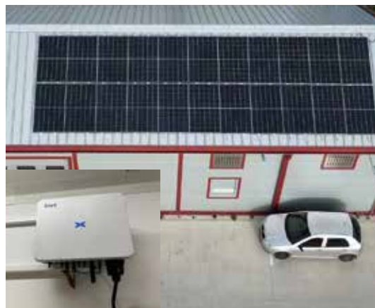
4kW Solar System in Slovakia (XG4KTR)
