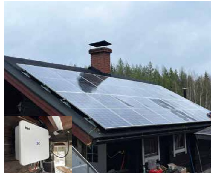
4kW Solar System in Finland (XG4KTR)
