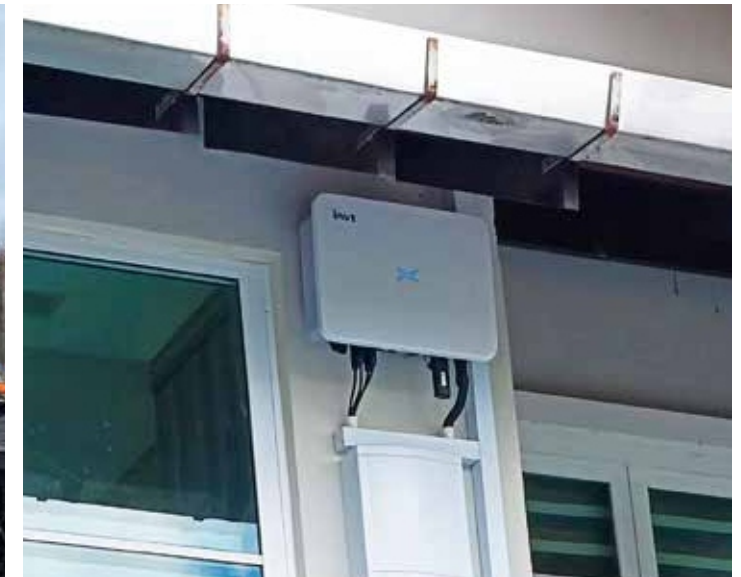
4kW Solar System in Malaysia (XG4KTR)
