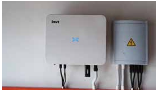
4kW Solar System in Malaysia (XG4KTR)
