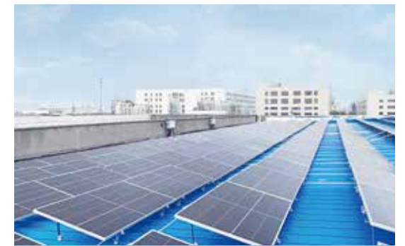
◆◆◆kW Rooftop PV Plant in Slovakia (XG◆◆KTR XG◆◆KTR)
