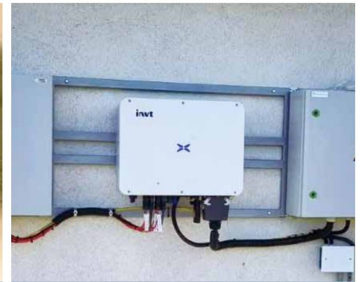
4kW Solar System in Serbia (XG4KTR)
