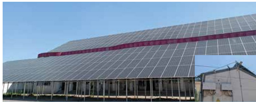
◆◆◆kW Rooftop PV Plant in Shanxi, China (XG◆◆◆KTR)
